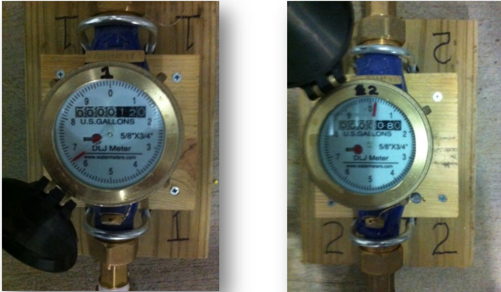
Figure 10. Two water meters purchased and installed on March 20 th , 2014 to measure pen wash down water additions to manure volume. Initial meters readings were 126.6 and 80.2 gallons for meter 1 and 2.
