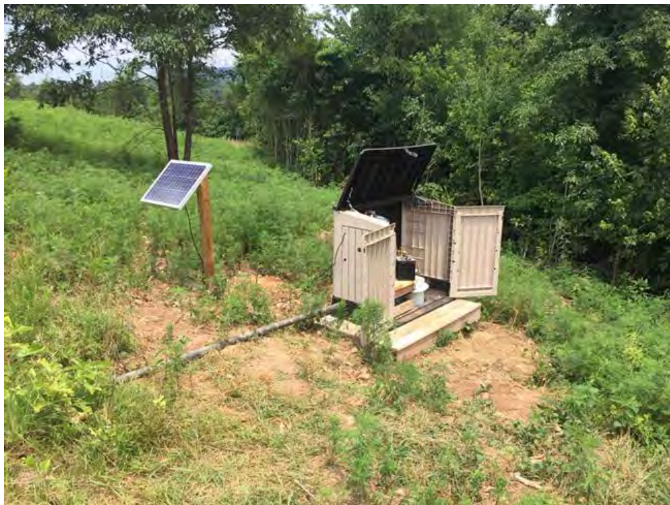
Figure 5. External view of interceptor trench flow monitoring equipment.
