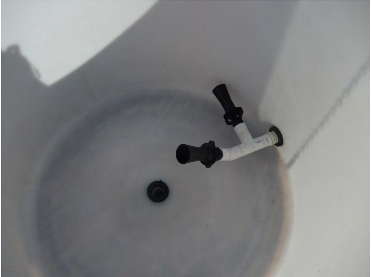
Figure S 2. Inlet nozzles inside the manure slurry collection tank, configured to mix manure slurry as it is pumped from holding pond 1.
